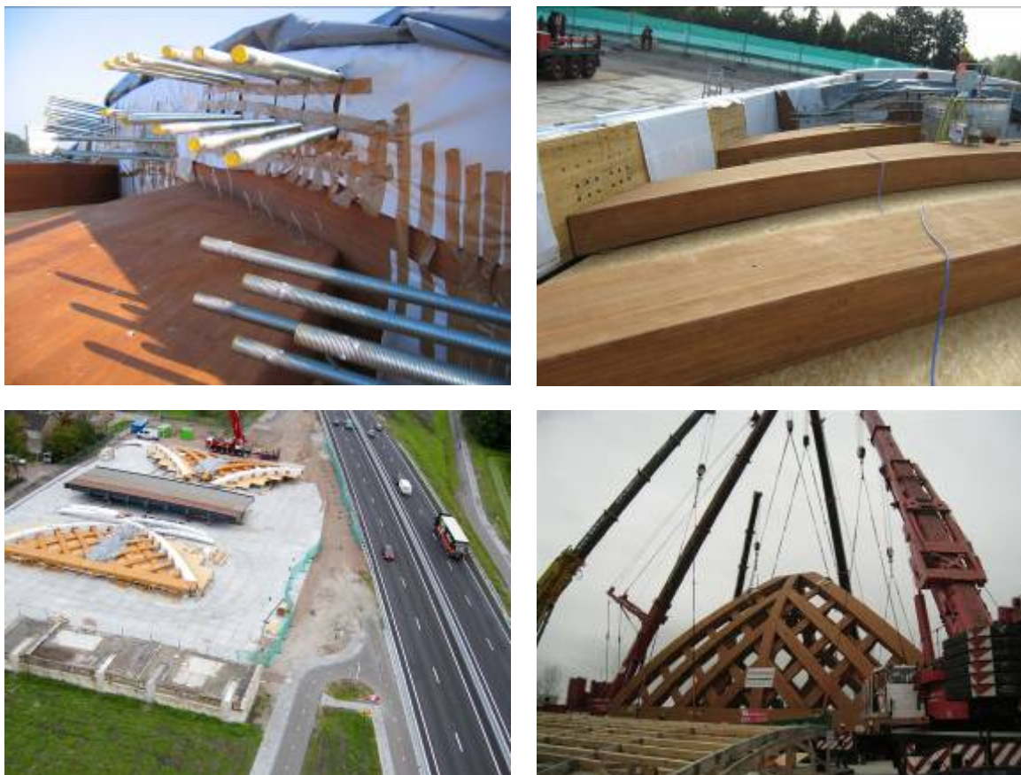
Figure 5: Assembling the elements of the bridge on a location near the high way A7 in Sneek. All parts are assembled with glued-in threaded rods, which have substantial metric studs to a girth of 48 mm. An important matter was the connection of the rod ends that were finally secured into the wood by way of injection with an epoxy glue
