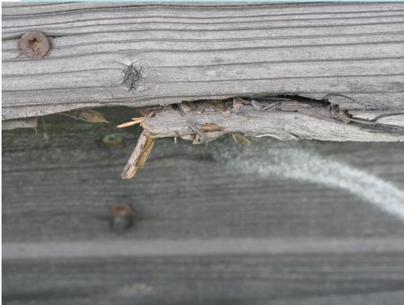
Example: Spot of slight decay
