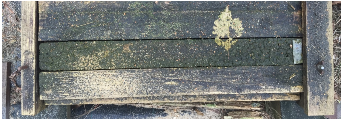
Figure 3: Surface of horizontal double layer specimens after 14 years of exposure. Formation of biofilms in artificial shade associated with superficial growth of algae.
