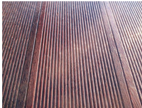
Figure 3: Bangkirai test deck, originally with 5 mm gaps totally closed up after being exterior exposed.
